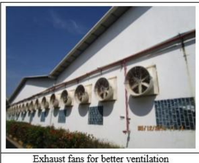
Exhaust fans for better ventilation
